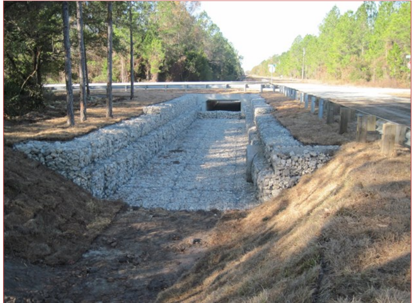
Gabion lining designed to prevent erosion
