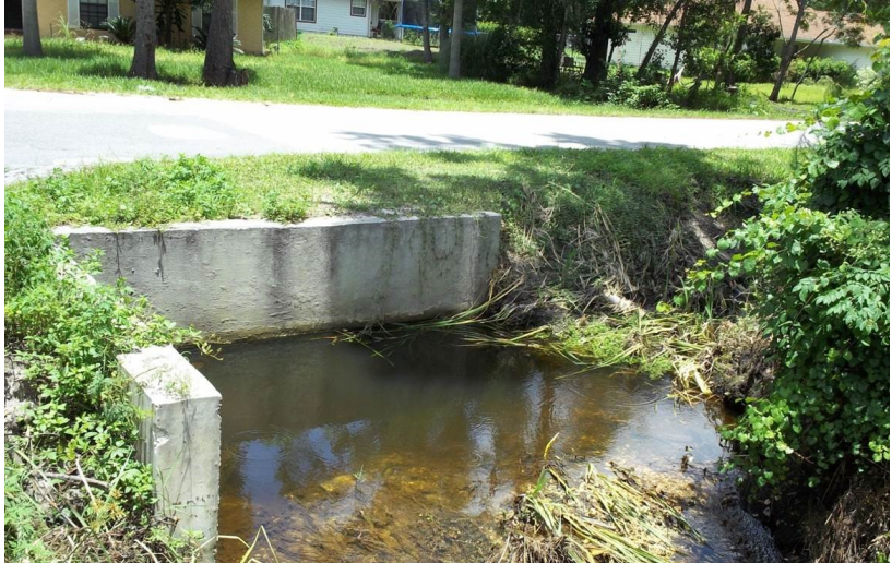
Baffle box designed to clean stormwater exiting the drainage basin
