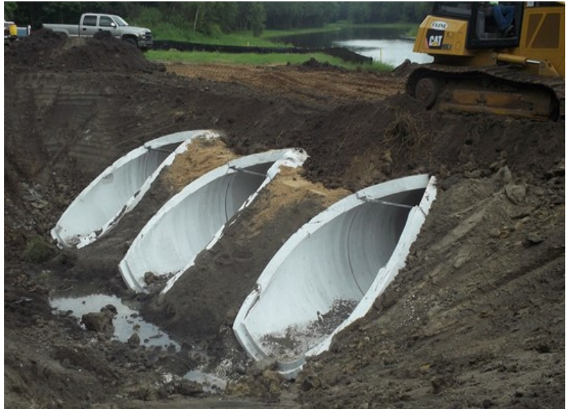
Reinforced pipes convey water flow from the Ashley Canal.
