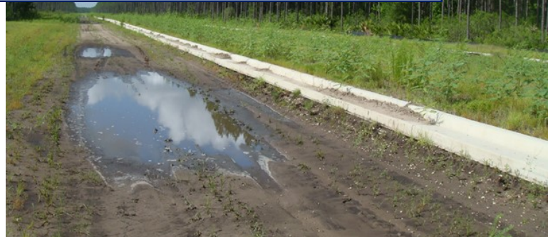
Graphic shows construction cross section for CR 223, a road that will connect CR 210 to Veteran's Parkway in St. Johns County.
